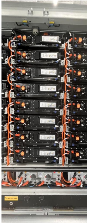
Figure 6-4-2 (6) Image of communication and power cables in Rack
