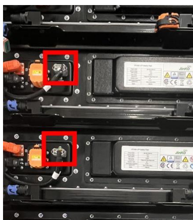
Figure 6-4-2 (2) Image of communication cable connector on HV BOX
