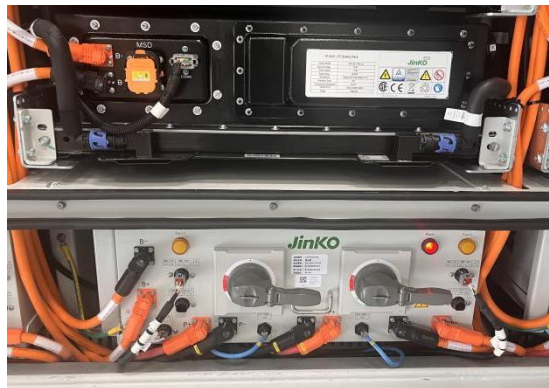
Figure 6-4-2 (5) Image of the communication and power cables between the PACK and the high voltage box inside the Rack.
