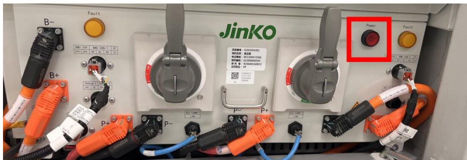
Figure 7-1-2 (4) HV BOX-DC 1500V power on
