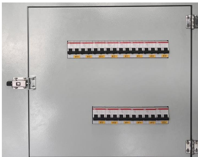
Figure 7-1-2 (2) Control Panel with switches of integrated cabinet
