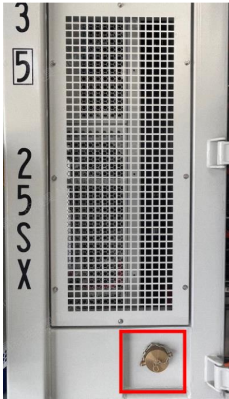
Figure 8-2 (10) Image of external DN65 water supply port for water fire fighting
