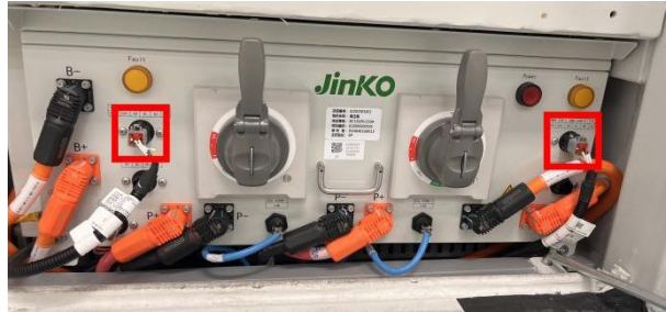
Figure 6-4-2 (3) Image of communication cable connector on HV BOX
