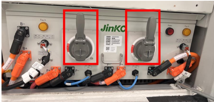
Figure 7-1-1 (1) HV BOX circuit breaker
