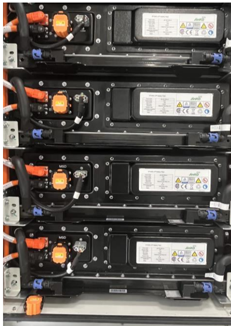
Figure 7-1-1 (2) Power cable connections
