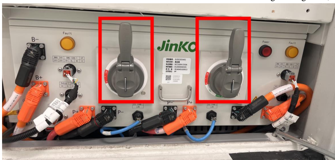
Figure 6-4-2 (1) Image of DC circuit breaker for high voltage box
