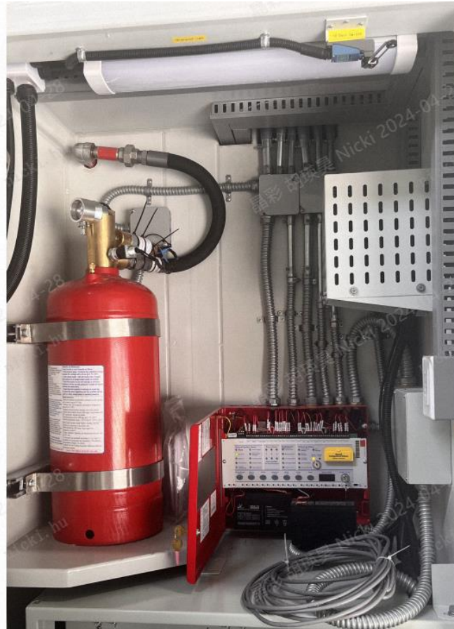
Figure 8-2 (6) Image of fire control panel and gas cylinde
