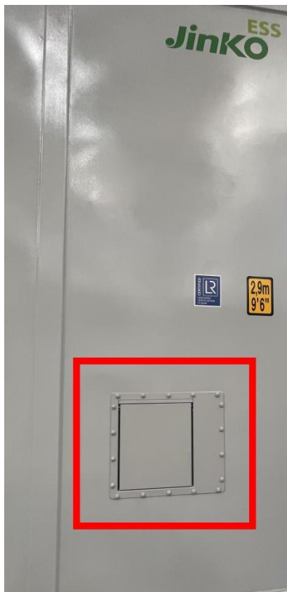
Figure 8-2 (8) Image of air inlet
